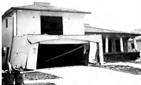
Photo 2. Severely damaged one- and two-story wood frame dwelling on Almetz Street in Sylmar District.
